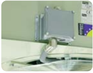
Outside connecting box
